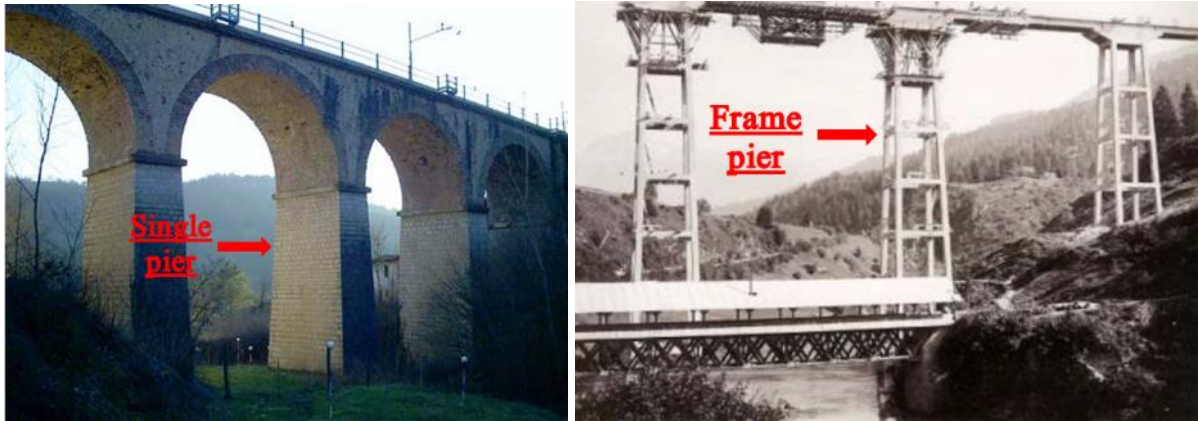
Figure 38. On the left, single piers – Source: [33]. On the right, frame piers of Ponte Vallesella, Belluno – Source: [34]
