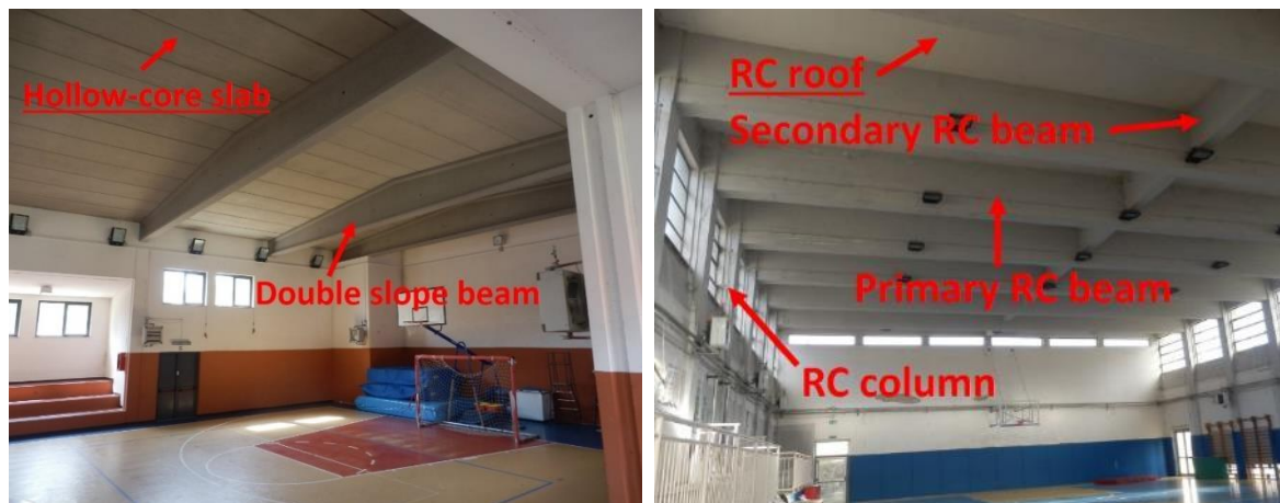
Figure 51. On the left, roof with hollow-core slab. On the right, RC roof – Source: [7]
