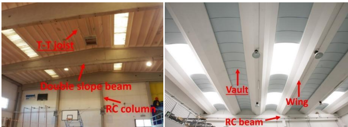
Figure 54. On the left, T-T joist elements – Source: [7]. On the right, roof with vault elements – Source: [39]
