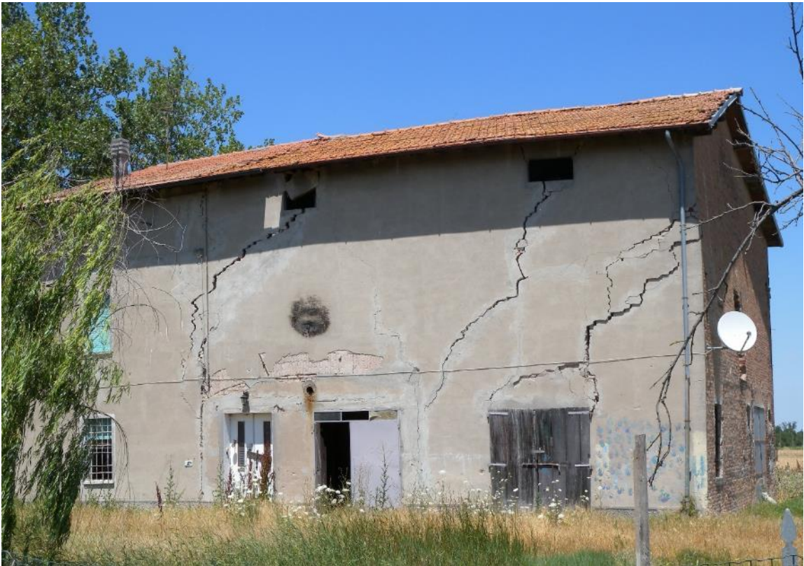
Figure 8. Cracks and masonry spalling on unreinforced masonry building - Source: [37]
