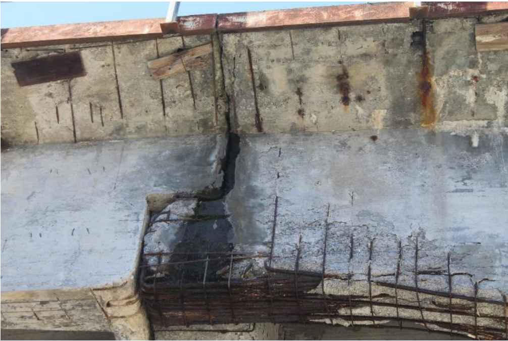
Figure 12. Spalling of RC beam and slab with leaching and corrosion of reinforcement, severe in the Gerber saddle - Source: [37]
