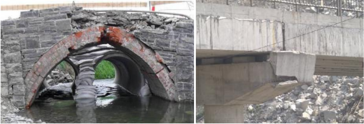
Figure 14. On the left, damage to the arch of Saby’s Road Bridge – Source:[46]. On the right, pier cap damaged – Source: [47]
