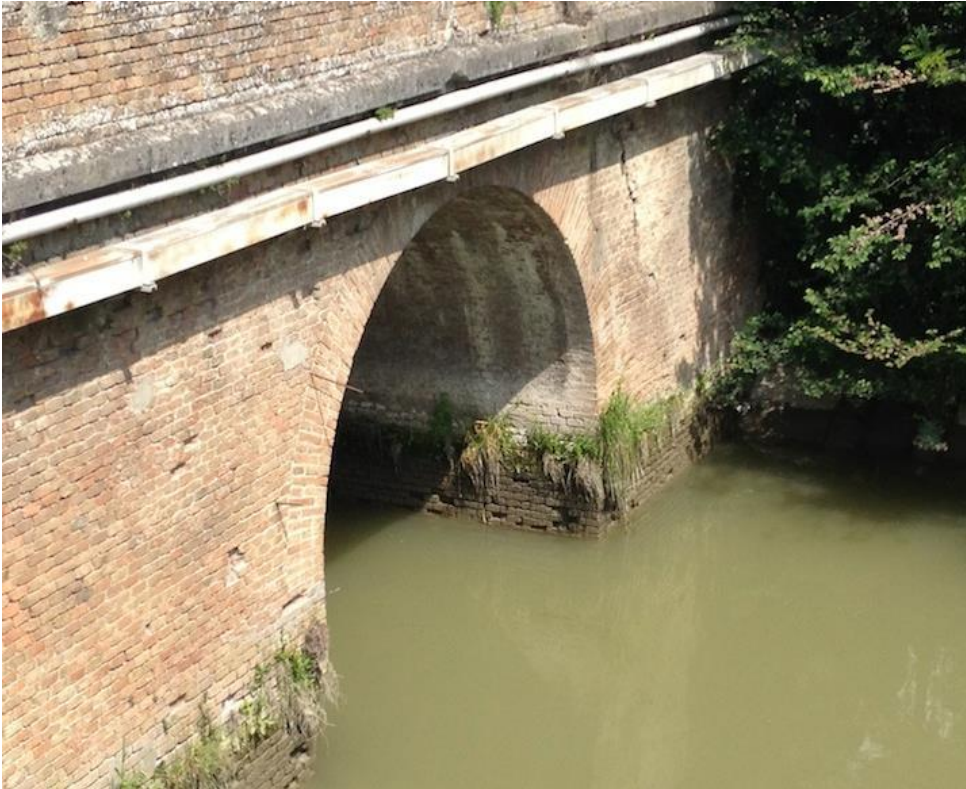
Figure 9. Crack on masonry arch bridge, with leaching and spalling - Source: [37]
