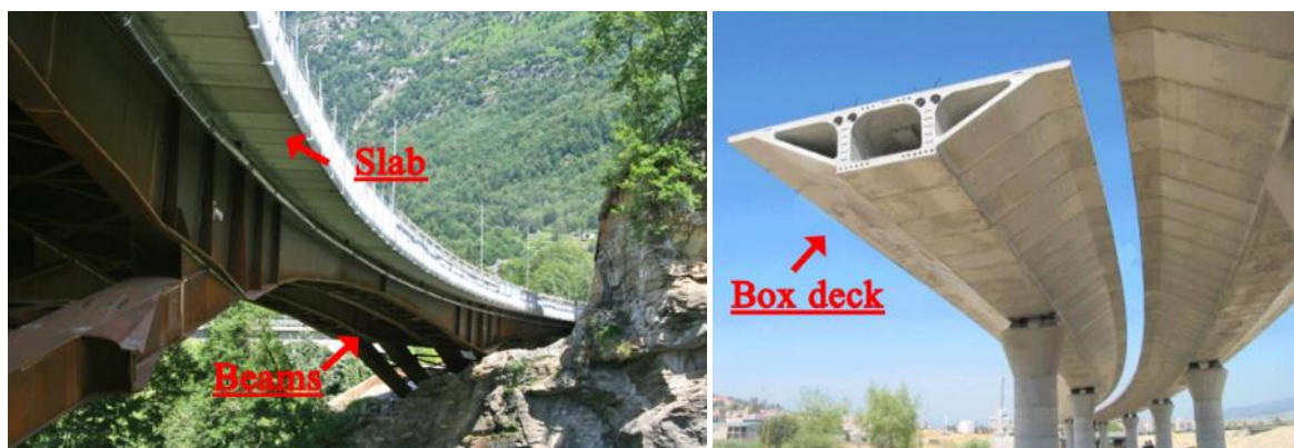
Figure 31. On the left, Ponte di Baceno (VB), with steel girders and reinforced concrete slab – Source: [22]. On the right, Autostrada SA – RC, viaduct with box deck – Source: [23]
