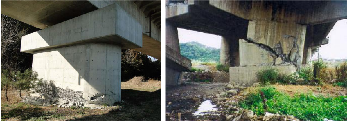
Figure 15. On the left, flexural break of the pier in the overlapping bar zone – Source: [48]. On the right, shear break and consequent overturning of a pier of Wushi Bridge, after Taiwan earthquake in 1999 – Source: [49].
