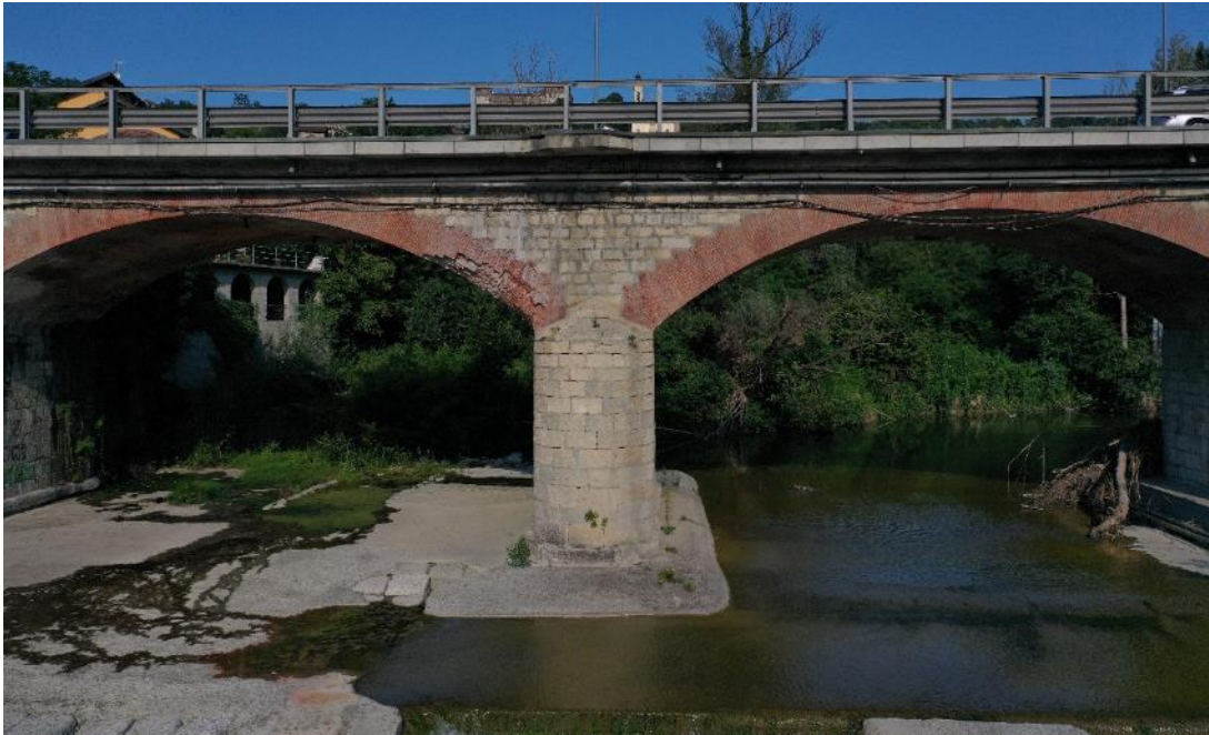
Figure 10. Masonry spalling on arch bridge - Source: [37]
