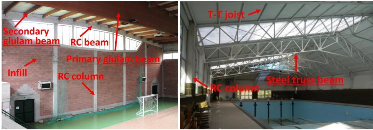
Figure 49. On the left, roof with glulam beam. On the right, roof with steel truss beam – Source: [7]
