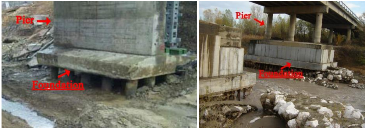
Figure 32. On the left, scouring of foundations - Source: [24]. On the right, scouring of foundation plinths: Ponte della Pedemontana – Source: [25]
