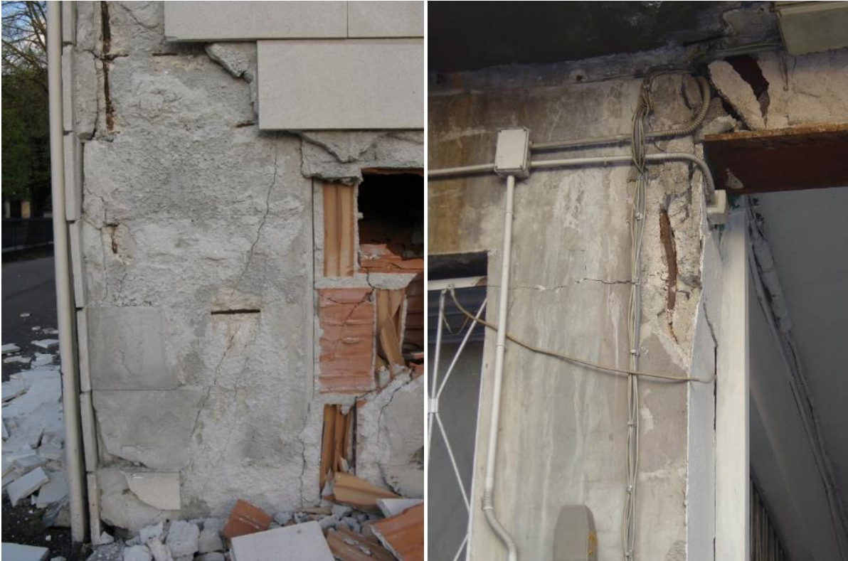
Figure 17. On the left, shear crack on RC column, with spalling, corrosion of reinforcement and debris from the collapsed infill and cladding. On the right, flexural crack on RC column, with spalling and reinforcement corrosion - Source: [37]
