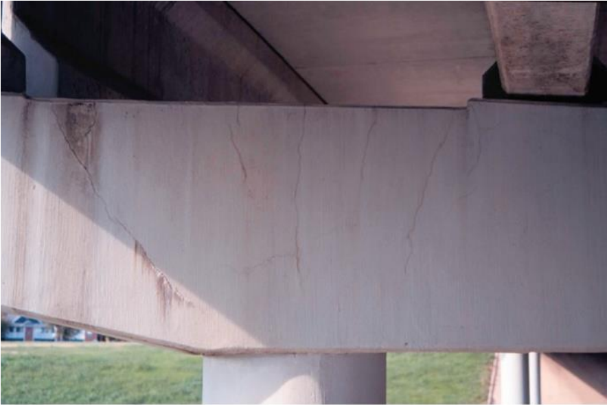
Figure 11. Pier cap with vertical flexural cracks over the column region and shear crack propagating from the girder – Source: [37]
