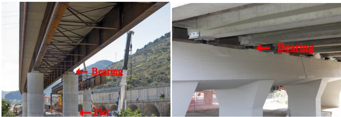
Figure 27. On the left, Viadotto Castagne – Source: [15]. On the right, identification of bridge bearings – Source: [16]
