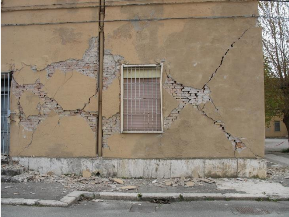
Figure 7. Shear cracks and masonry spalling on the façade of a residential unreinforced masonry building – Source: [37]
