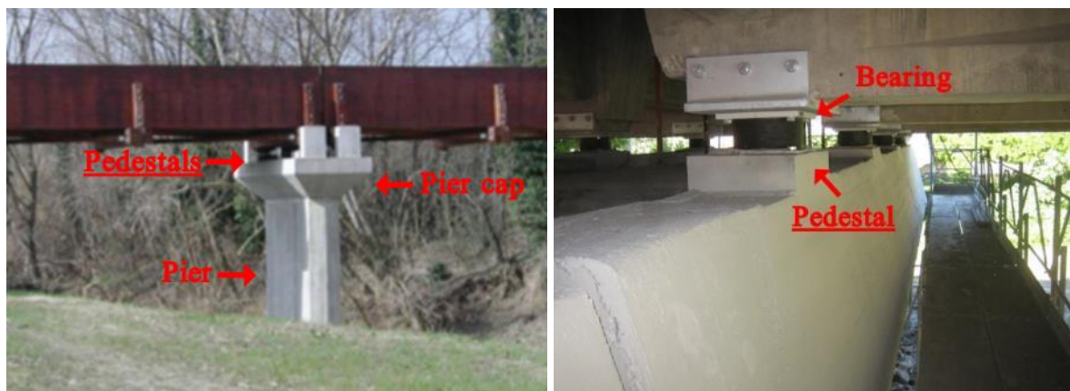
Figure 37. On the left, bridge pedestals of Pian del Bruscolo cycle path - Source: (Rossi, 2014). On the right, identification of bridge pedestals – Source: [16]
