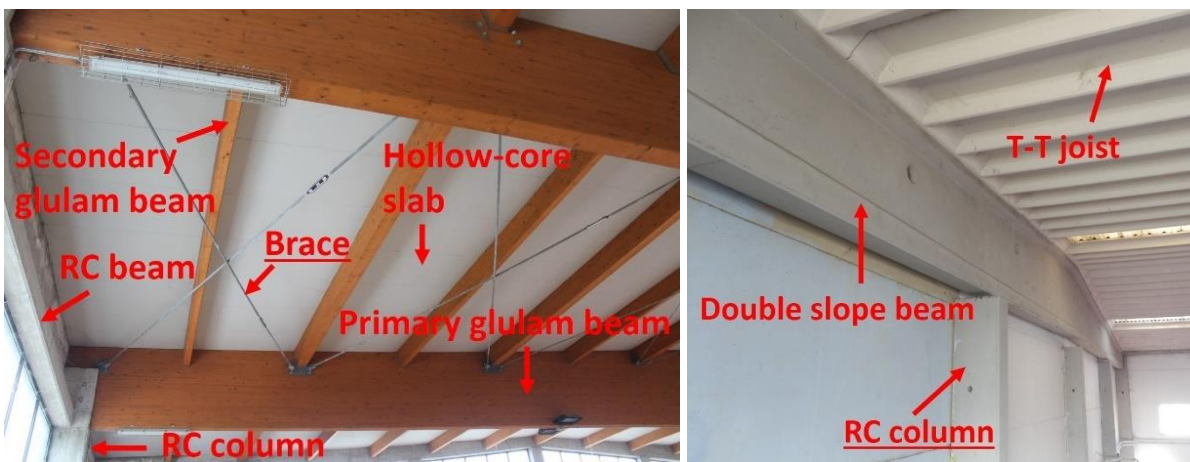
Figure 50. On the left, brace in roof plane. On the right, RC framework elements – Source: [7]
