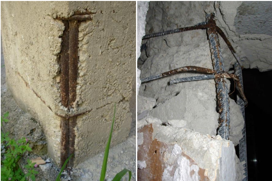
Figure 16. On the left, spalling and reinforcement corrosion in RC column. On the right, spalling in RC column, with corrosion and deformation of steel reinforcement - Source: [37]
