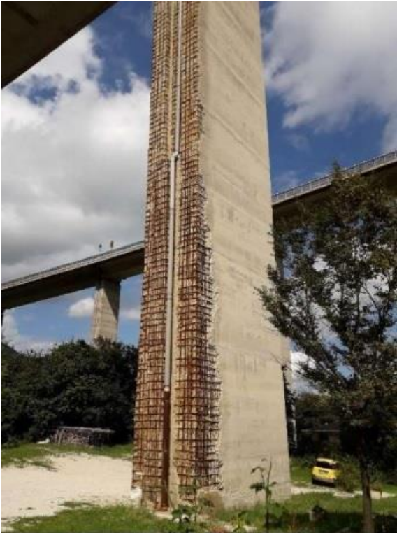
Figure 13. Severe spalling of bridge pier with reinforcement corrosion – Source: [45]
