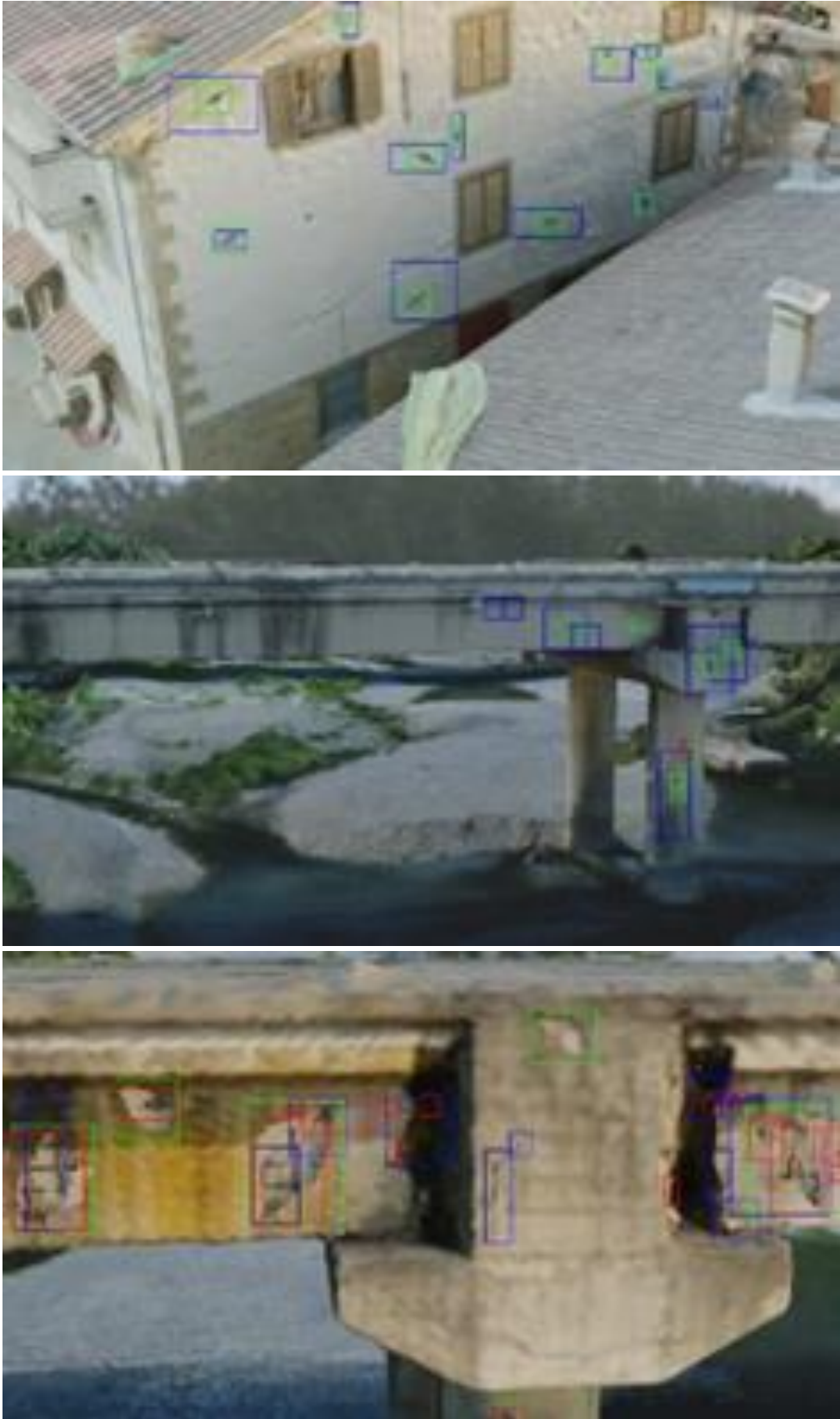
Figure 23. Some examples of the final rendering with bounding boxes (different colours mark different type of damages)
